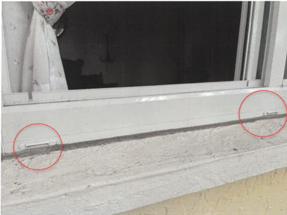
Figure 8: Typical drainage weepholes (red circles). Photo used with permission.
