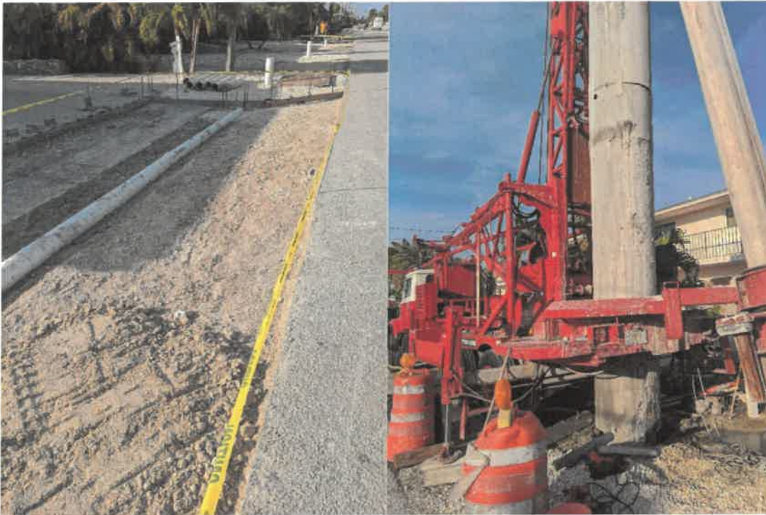
Key Colony Beach 10 th Street Stormwater work from 2022 as an example of proactive measures.
